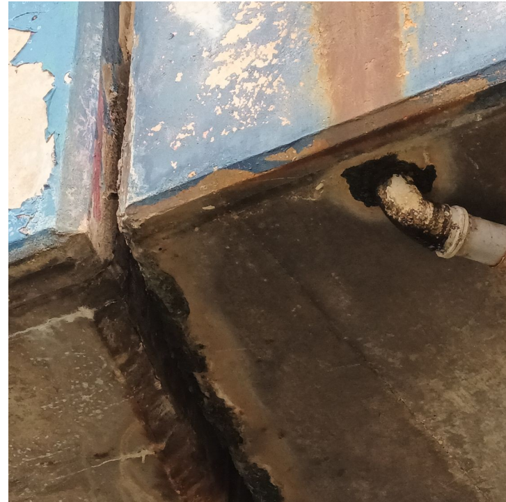
Figure 6: Detail of expansion joint on western face showing separate drainage from deck
