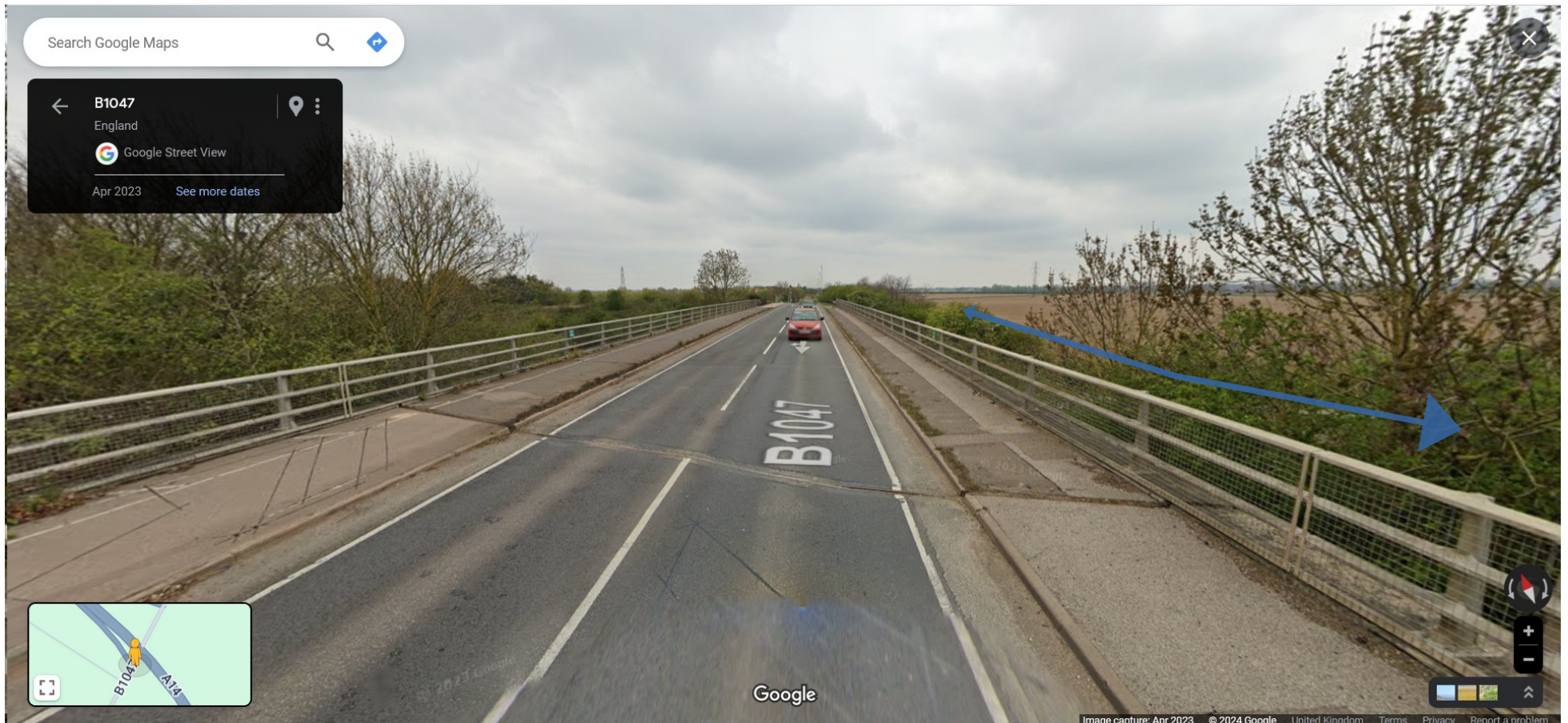
Figure 10: View of J34 looking north showing lack of street lights on bridge
