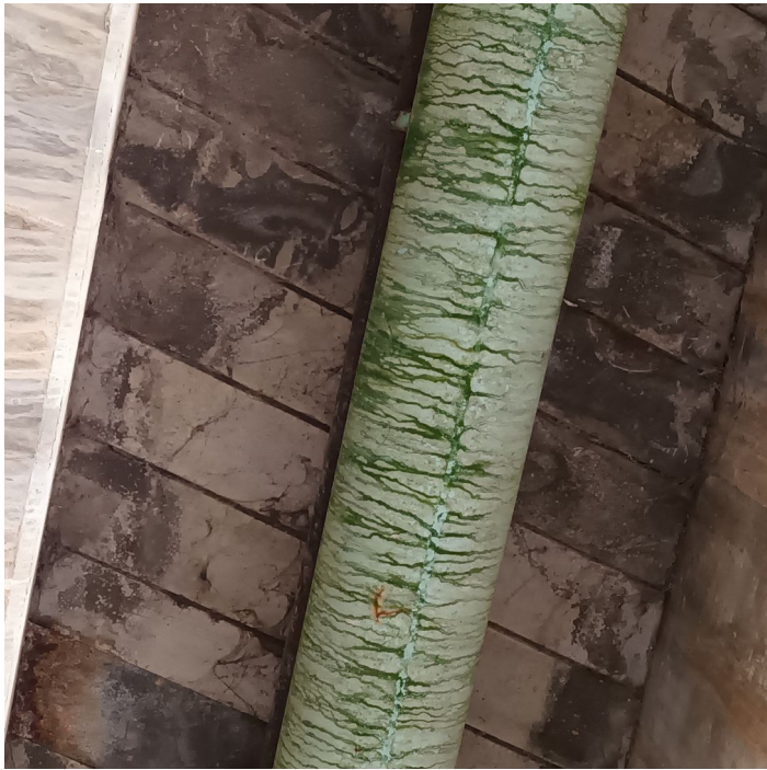
Figure 7: Detail of underside of central reservation showing pipe and additional crevices
