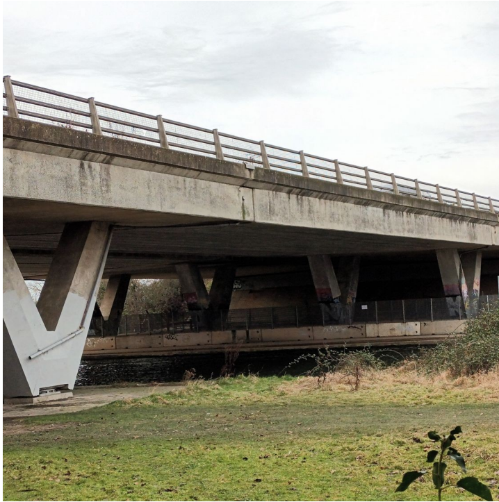
Figure 1: View from east of A14 crossing. Note expansion joint in bridge deck
