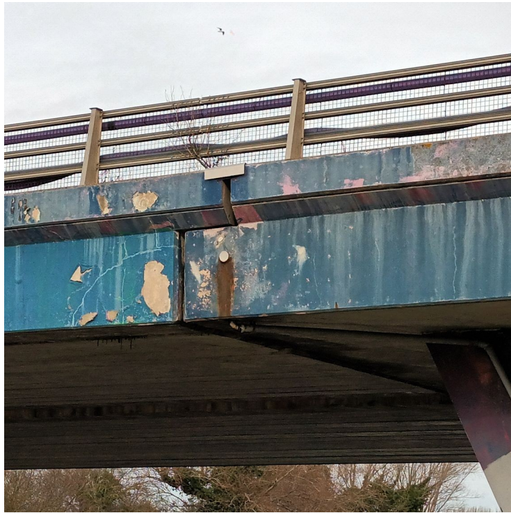
Figure 5: Expansion joint on Western face showing willow growth into cracks
